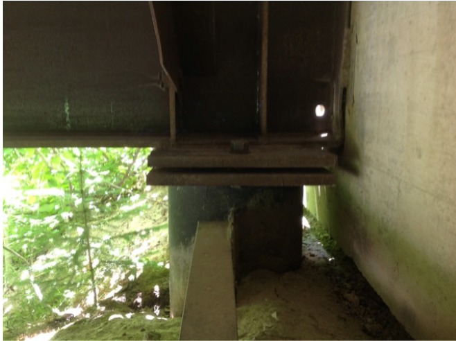
left upstream bearing
