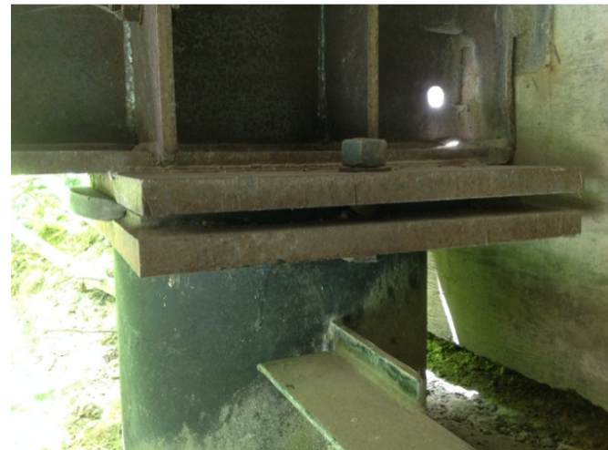
left upstream bearing
